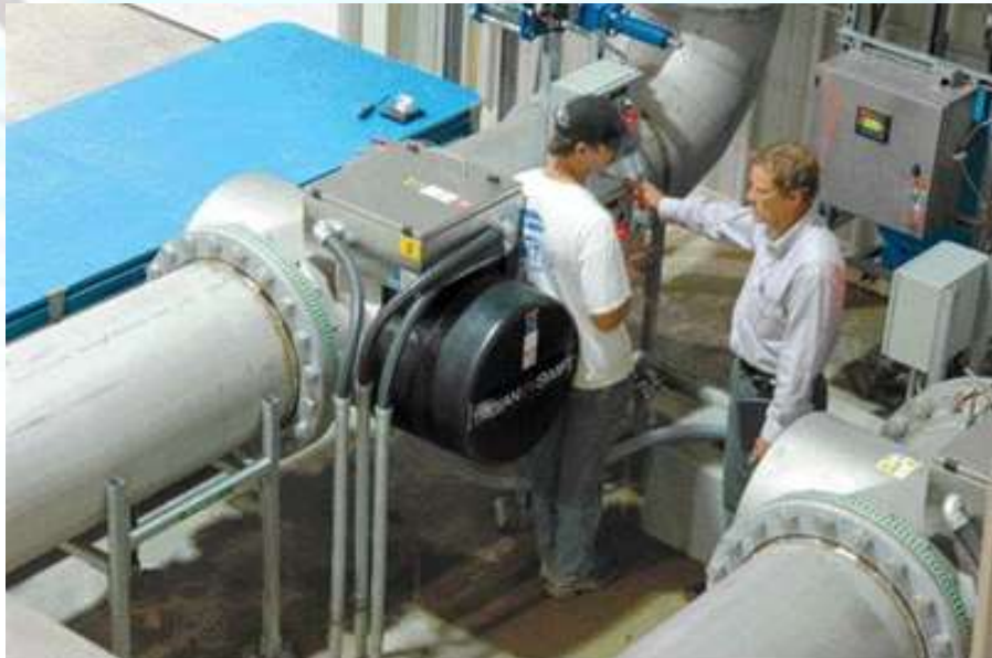
Arrow Creek Ultra Violet Disinfection Equipment
